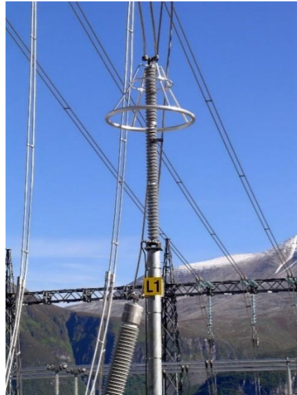
Plate 5.7 – Typical HV Surge Arresters Image: ©ABB
