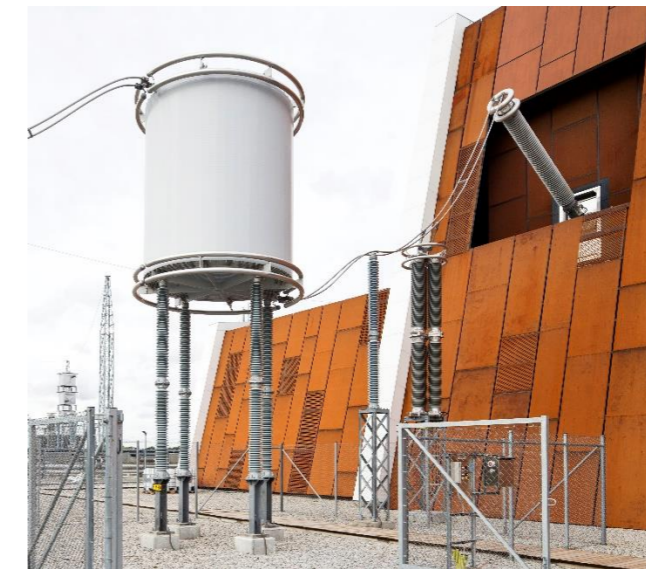
Plate 5.19 – Typical Phase reactors (outdoor) Image: ©GE
