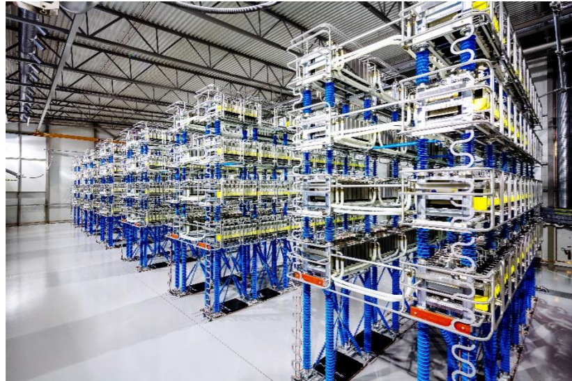
Plate 5.21 – Typical Valve Hall with stacks of Power Modules Image: ©GE
