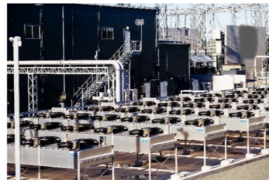
Plate 5.23 – Typical Outdoor Heat exchangers Image: ©GE
