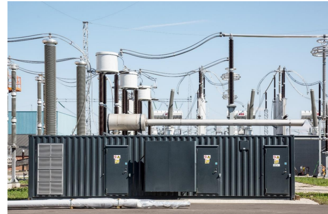
Plate 5.13 – Typical Diesel Generator Image: ©ABB
