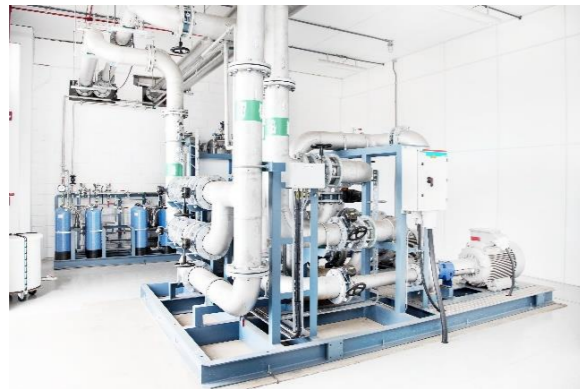
Plate 5.22 – Typical Water Pumping Station Image: ©ABB
