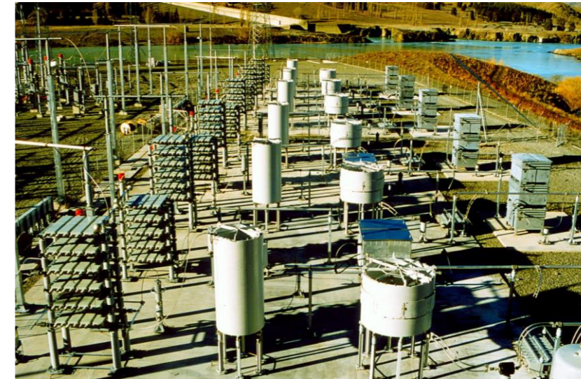
Plate 5.11 – Typical AC Switchyard Harmonic Filters Image: ©ABB
